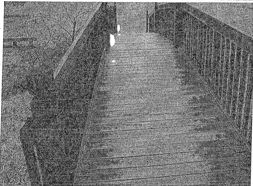
PHOTO #8 The wood footbridges at the footpaths also range from fair to good condition. This bridge is deflecting to the left side. We have scheduled bridge replacement in the next couple of years.
