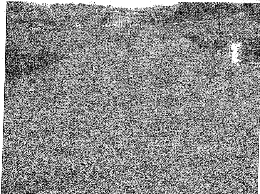
PHOTO #3 The asphalt footpaths range from new to fair condition. Any tripping hazards on the trails should be mitigated. Path lighting is new, but six of the lights were out of service.
